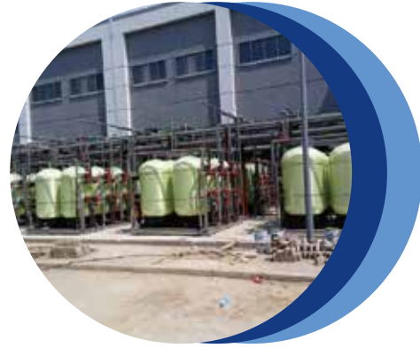
High-Purity Water Project in Jiangsu Province's Electronics Industry
